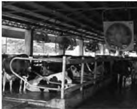
A typical Fans and spray arrangement
